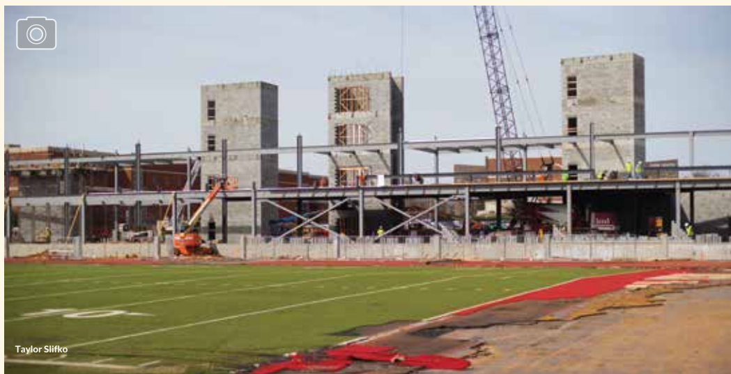
Crews continue work on Governors Stadium in March as the renovation begins to take shape against the campus skyline.
